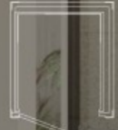
Manually operated door
